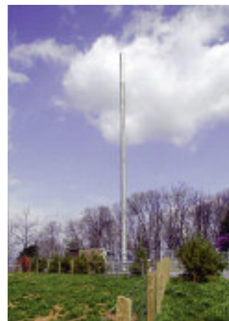
Slim, unobtrusive monopole, Rockbridge County
