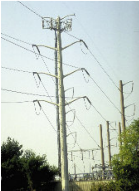
Co-located on transmission tower
