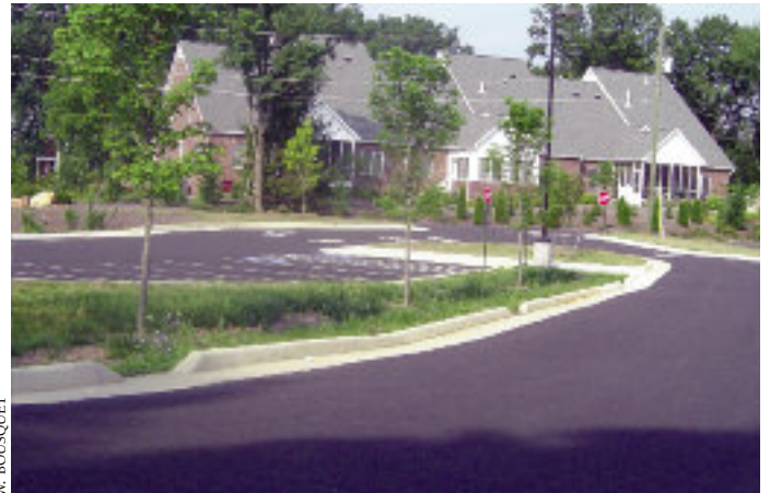
Curb inlets help runoff flow into tree islands at McSwain Elementary School, Staunton.
