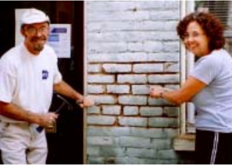
These board members do more than attend meetings. James Flory, an accomplished stone mason, and Faye Cooper repoint bricks on VCC's historic office building.
